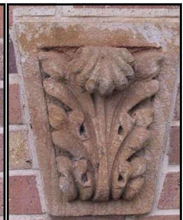
The right hand gatepost containing the keystone from the ground floor window
